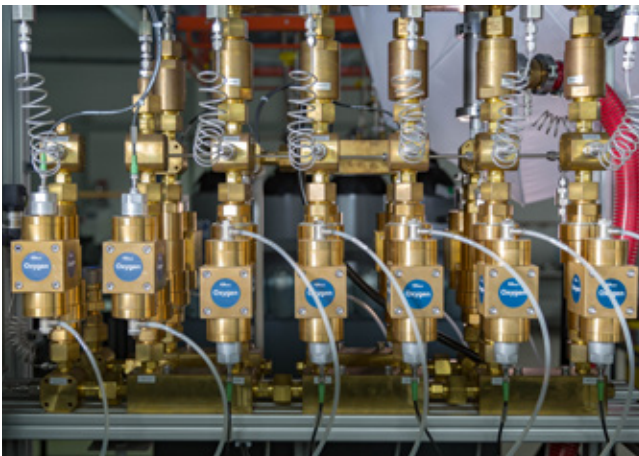
Example of a technical gas plant with TV17 valve assemblies:
