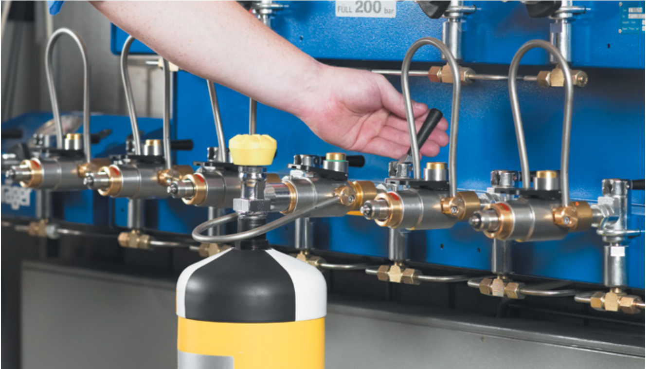
Existing BA cylinder filling rig after it has been upgraded to using the CLICKMATE® TW154
